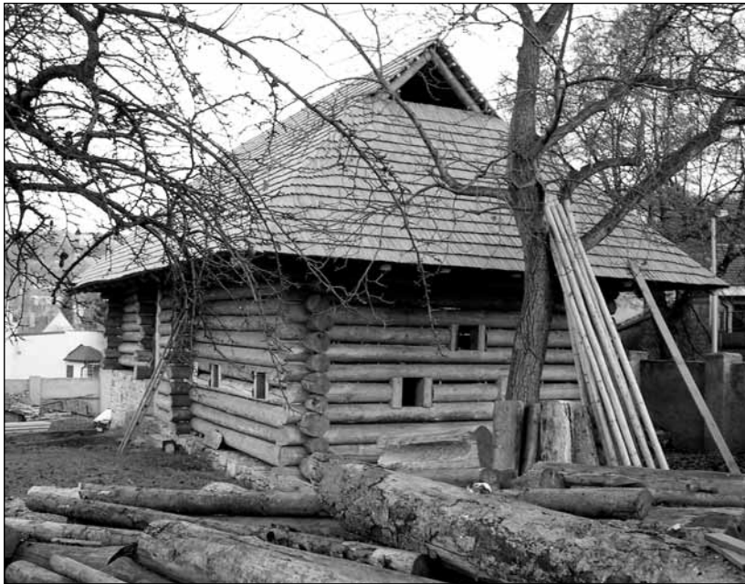
Fig. 28 Building of a three part house B1: look at the gable and yard eave walls of the finished rough building. ■
