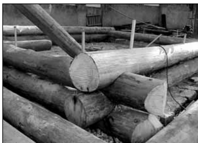
Fig. 24 Building of the three part house B1: detail of corner joints of the log construction with irregular ends of logs. ■
