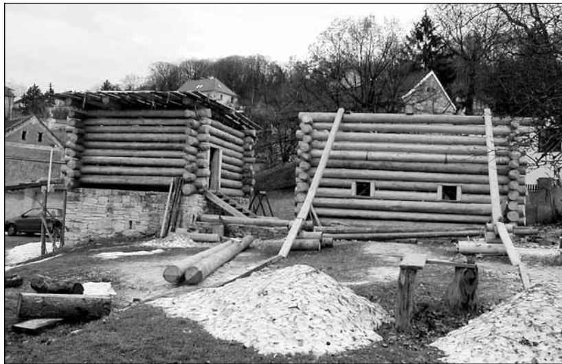
Fig. 23 Building of a three part house B1: log built hall on the right, on the left lower storage space with stone walls and upper bedroom with log constructed walls. ■
