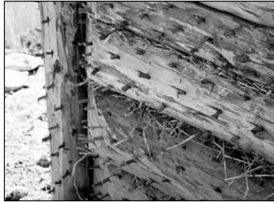
Fig. 17 Experimental building of structure B7: detail of the wall prepared for daubing. ■
