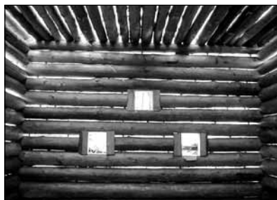
Fig. 26 Building of a three part house B1: interior of the hall with pyramidal organisation of windows in the gable wall. ■
