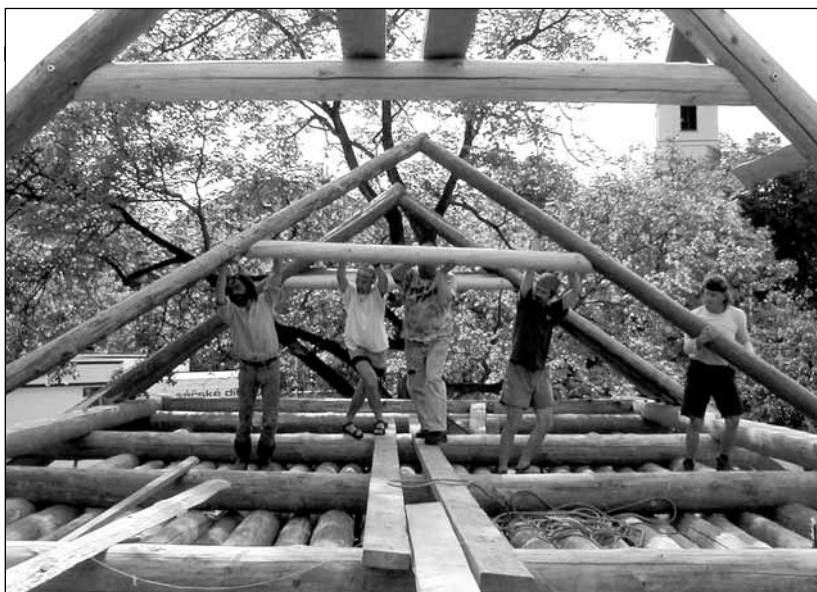
Fig. 25 Building of a three part house B1: erecting the rafter roof frame. ■
