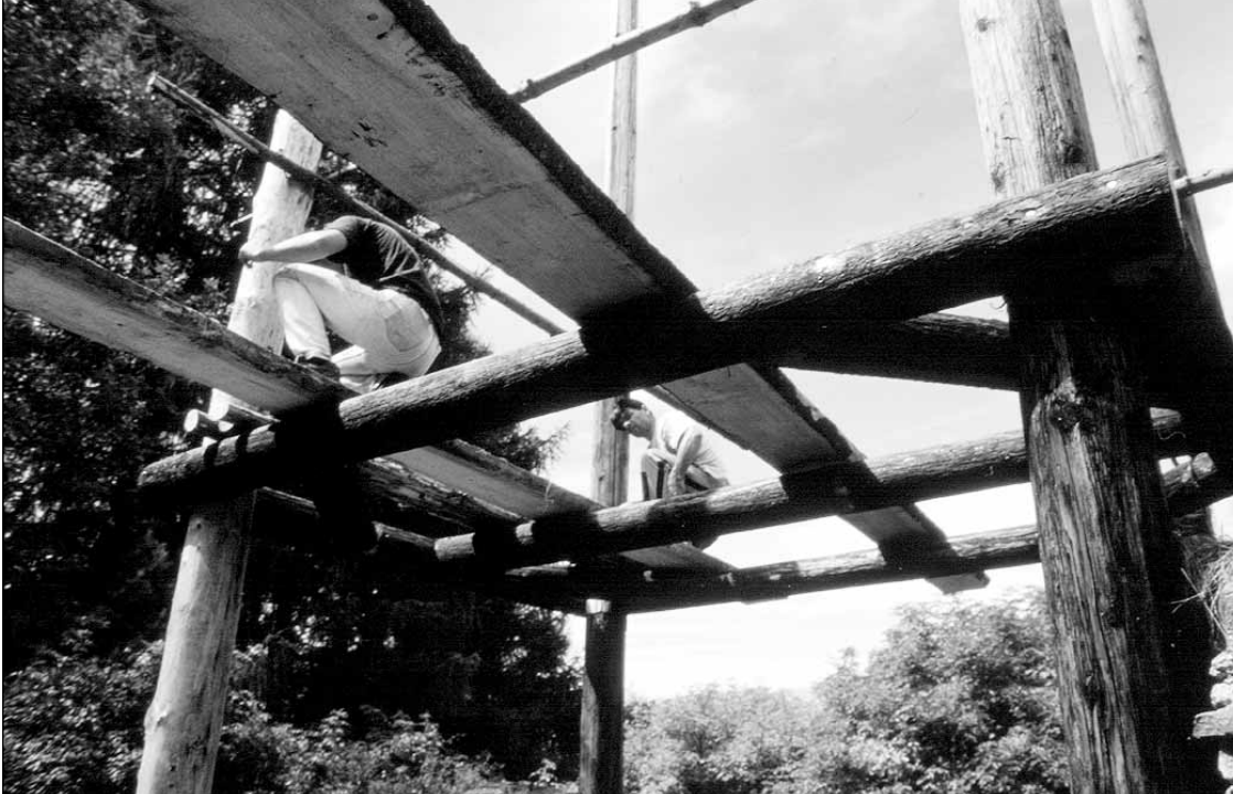
Fig. 2 The tower at the stage of a finished rough construction in the summer of 2003. ■
