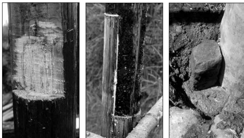
Fig. 4 Cleared and filled in area of rot at the joint of a post and rung. ■ Fig. 5 Extension of the damaged ends of posts with overlapping joint. ■ Fig. 6 Reversible fitting of a post into concrete. ■
