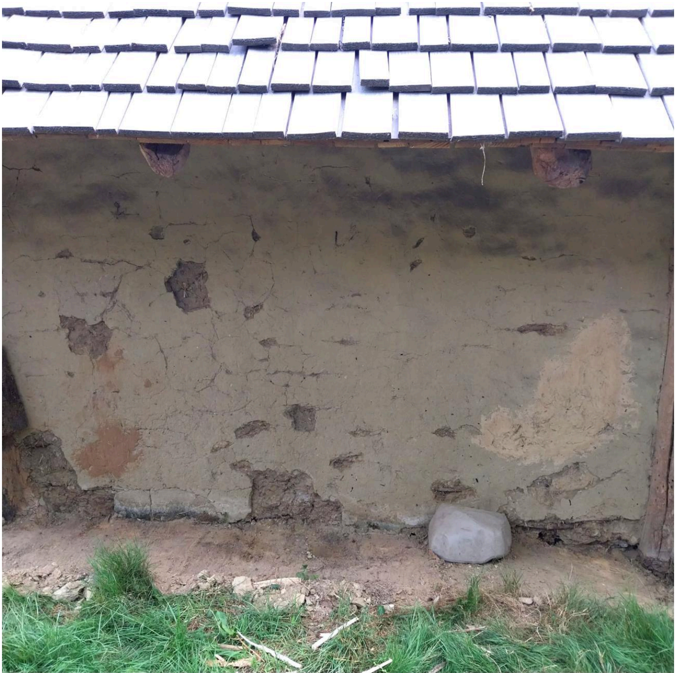
FIG 4. WALLS OF THE ROMAN BUILDING BEFORE REPAIRING. PHOTO BY AUTHORS
